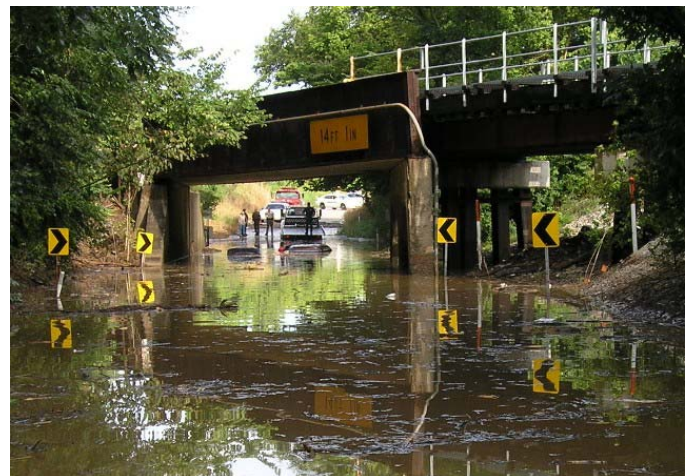
The Signal Hill Fire Dept. rescue at a flooded viaduct in St. Clair County after a storm on August 14.
