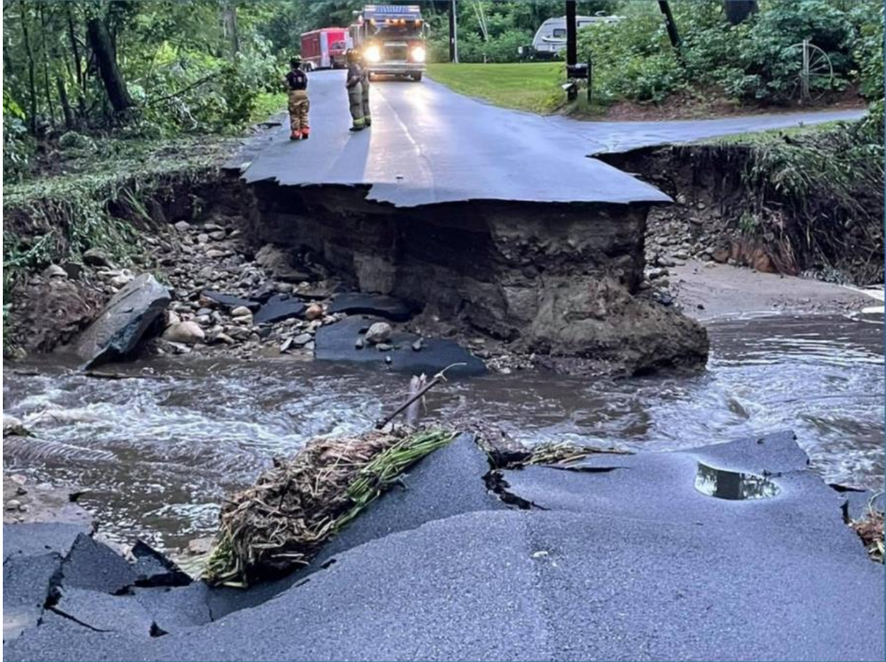
Road washout in Belchertown, MA (Photo: Belchertown Fire Department)
