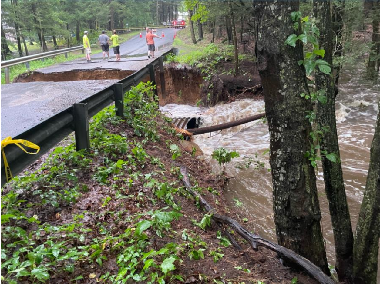
Road washout in Ashford, CT (Photo: Tom Borgman, Ashford Fire Department)
