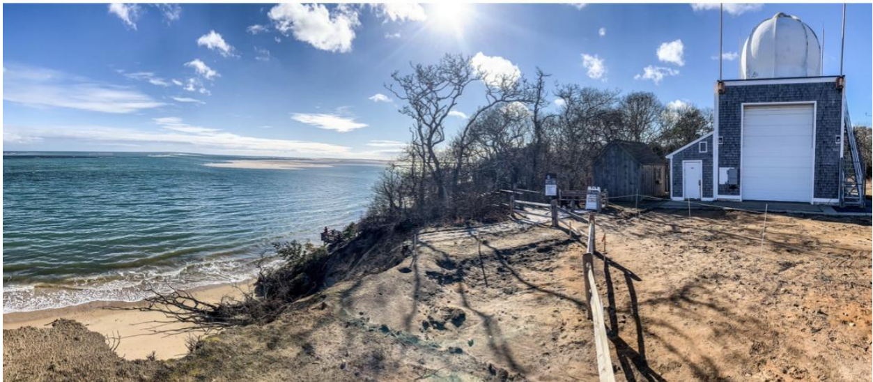
View of the Chatham Upper Air Station showing erosion of the bluff. (Photo: Bryce Williams)
